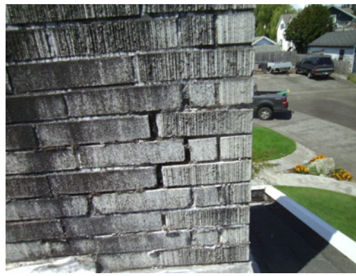
Upper chimney mortar deterioration
