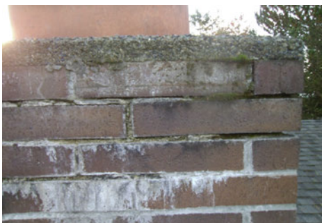
Deteriorated chimney brick
