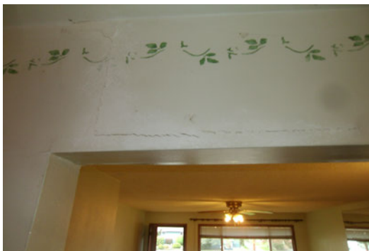
Interior wall fracture
